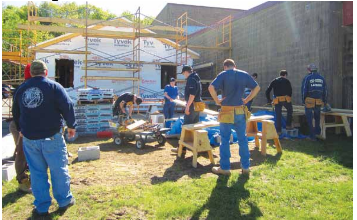
Tri-County RVTHS has partnered with the Town of Franklin to build a home as part of the town's affordable housing program. Guided by their instructors, juniors and seniors from the Carpentry, Electrical Wiring Technology, and Plumbing and Hydronic Heating Career Programs are currently working on construction of the house, which is scheduled to be completed by June 2015.
